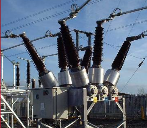
Dead Tank DT1-145 kV
